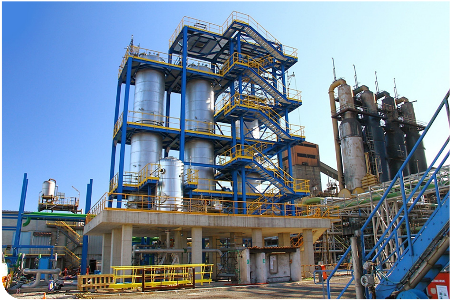
A new water distillation column at ArcelorMittal Fos-sur-Mer has reduced H 2 S levels.
